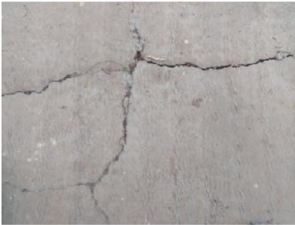
Fig. 7. Original Image of Road Crack.
