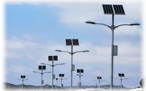
Figure 2: Solar panels on parking lights
