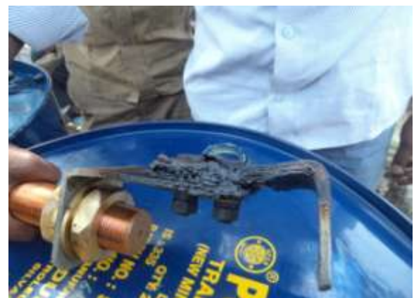
Figure 14- Damaged bushing clamp
