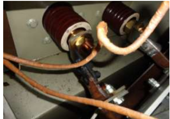
Figure 13- Faulty portion of bushing
