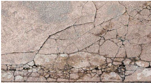
Fig. 2. Non-Structural cracks (gharpedia.com)
