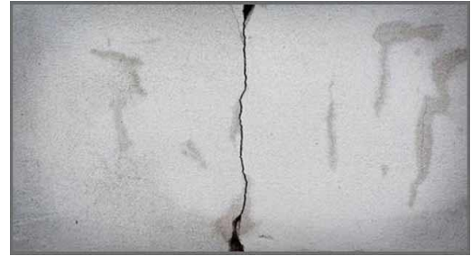
Fig. 4. (a) Medium crack (1-2mm) (constrofacilitator.com)
