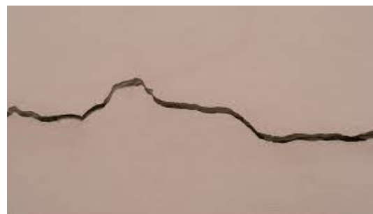
Fig. 5. Wide crack (>2mm) (loveproperty.com)
