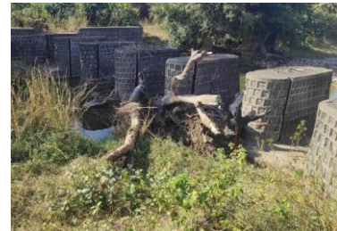
Fig. 2. Tree trunks and debris accumulation across the channel during flood season.
