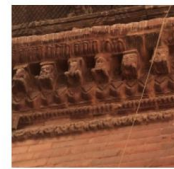
Lions Head Exposed on Cornice
