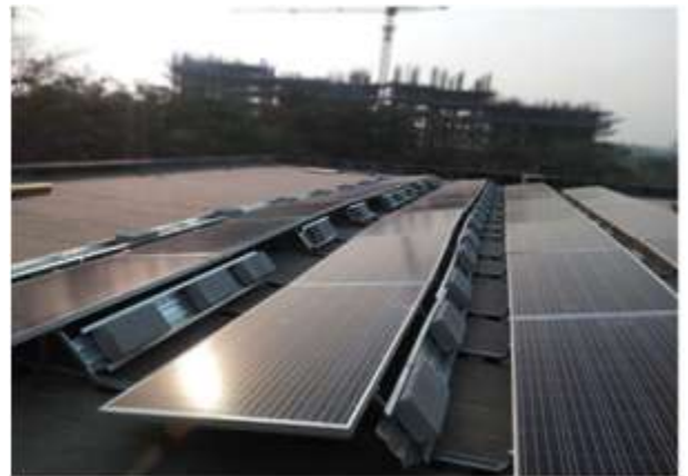
Figure 2: Solar PV Plant on rooftop of NCB-H
