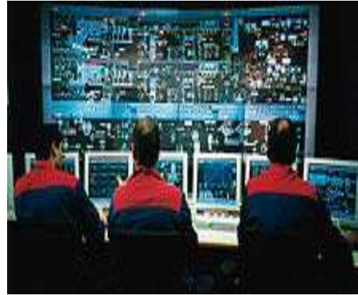
Figure 3 a DCS Control Room
