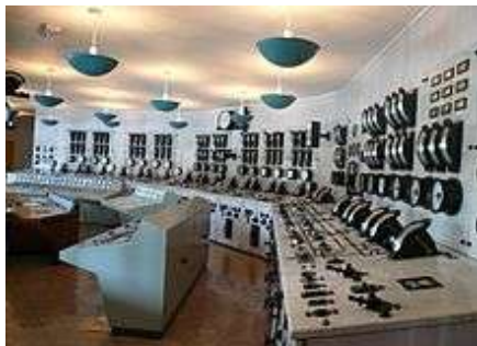
Figure 2 a Pre-DCS/SCADA Era Central Control Room
