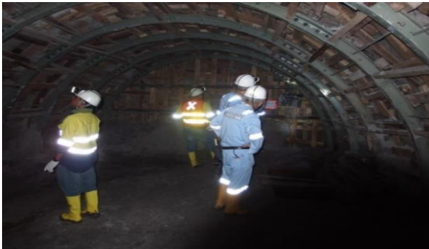
Fig. 11. Steel arch support
