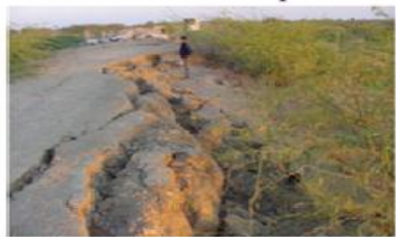
Embankment Failure - Bhuj Earthquake, 2001
