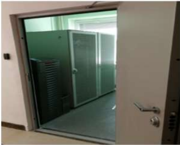
Fig. 2. Security door server, data, network center
