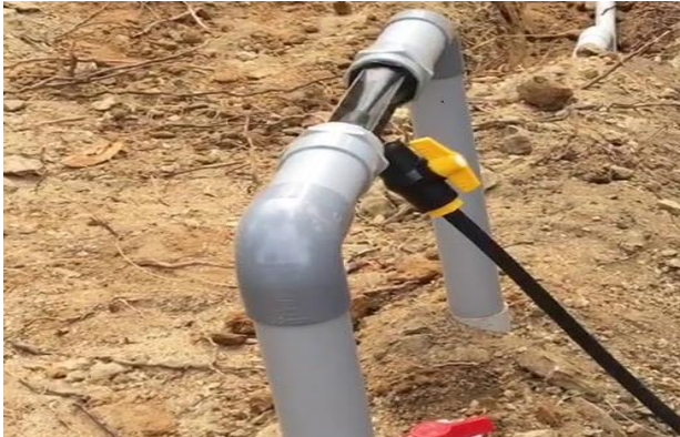
Figure.3. Pipe connected to submerged pump
