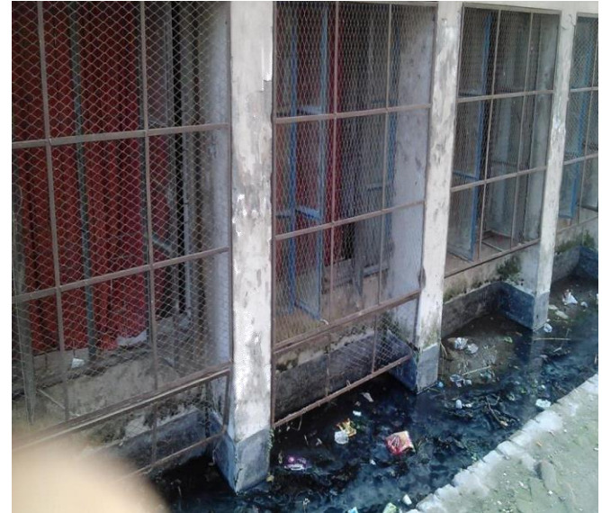
Fig. 12. Plumbing hazards in Mirpur
