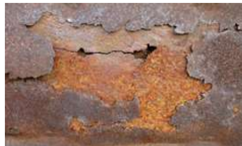
Fig. 4. Corrosion effect in boiler[16]
