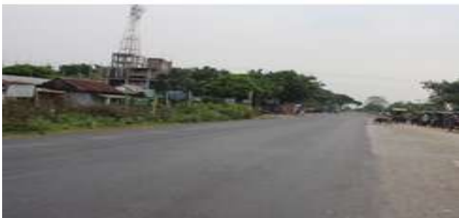
(a) No lane separated marking.
