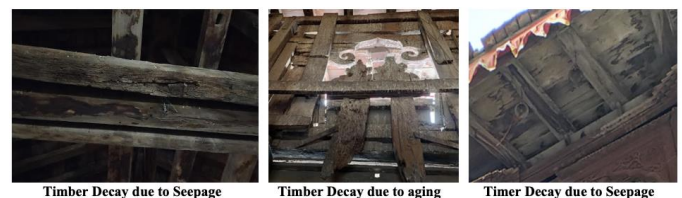
Fig. 7. Status of Timber
