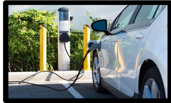
Fig. 5. Electric Charging Setup
