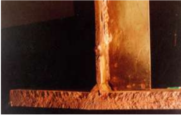
Figure 2: Girder flange fracture from Cherokee County, Iowa Bridge.
