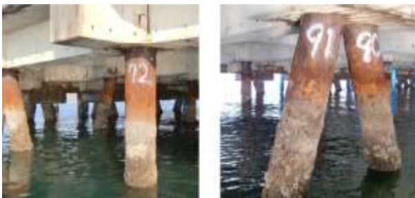
Figure 5: Corrosion-damaged pipe piles at an offshore pier (Xiao C. (2011) [22]).
