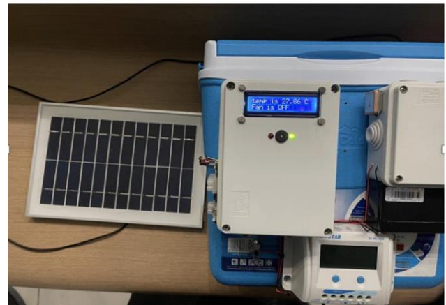
Fig.13. Temperature Monitoring System
